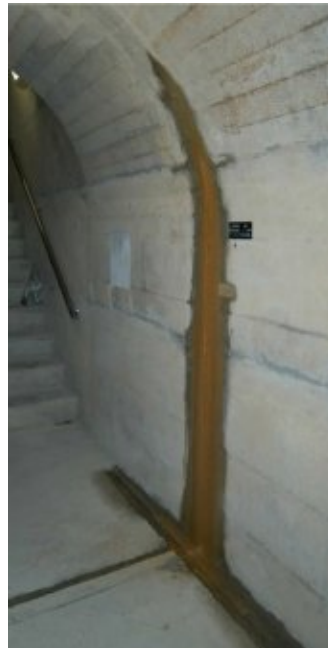
4) Leak prior to RADCON Formula #7 injection
