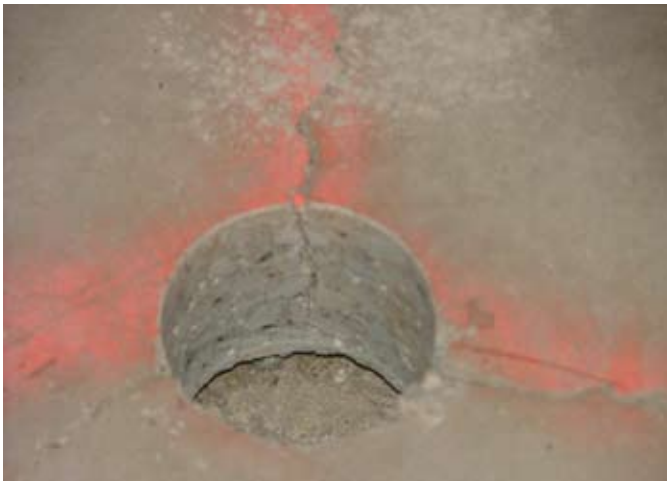
Fig. 1: After sounding with a hammer or other techniques to determine approximate locations, the delaminated area is verified with core-drilled holes
